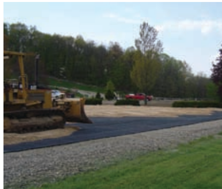
An inside look at the EquiBase™ Arena Systems Int'l. installation in the jumper ring at Old Salem Farm.
